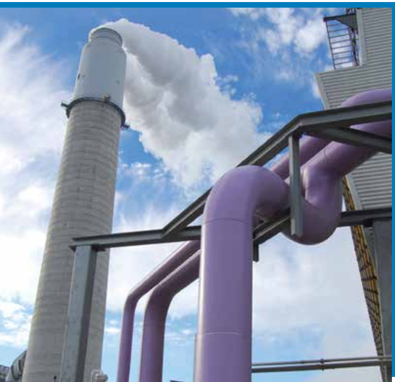
Reclaimed water is used at Plant Crist to operate the scrubber system, which reduces air emissions.
